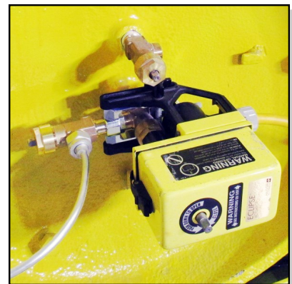
IV-810 with emergency shutoff actuator on a ton container with flexible connector.
